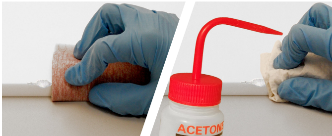
3. Sand with wooden block (N) and sandpaper P500 (D) only on the surface near the chipped area, then remove dust and clean the surface with acetone or alcohol.
